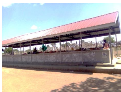
Figure 6: The Market shed constructed with a very narrow corridor.
