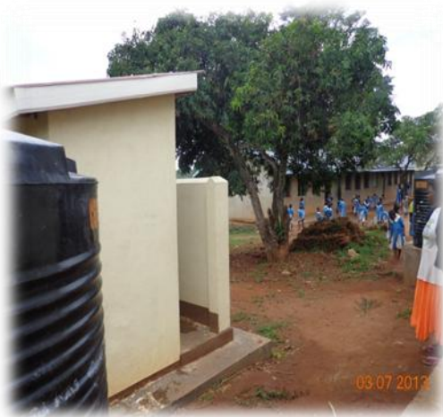
Completed two stances latrine under SFG for girls in Oweko p/s Completed latrine in Nyapea girl's primary school
