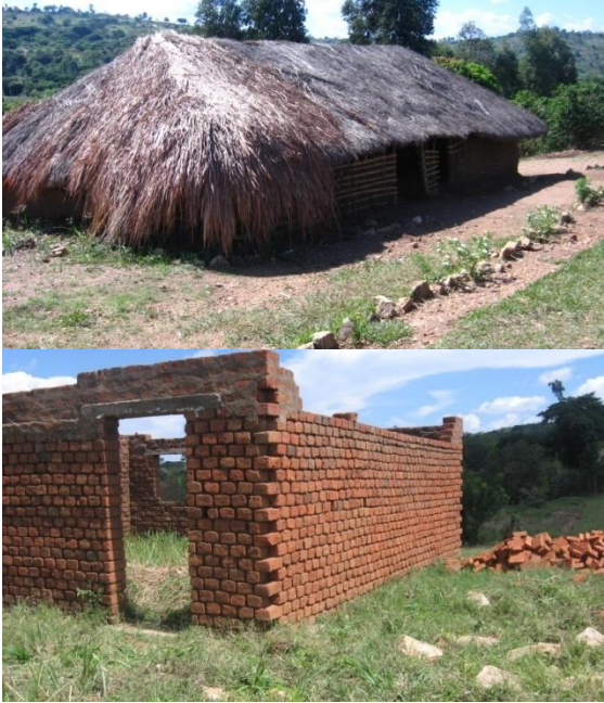
A classroom block in use (above) and a parents block under construction in Athele P/s.
