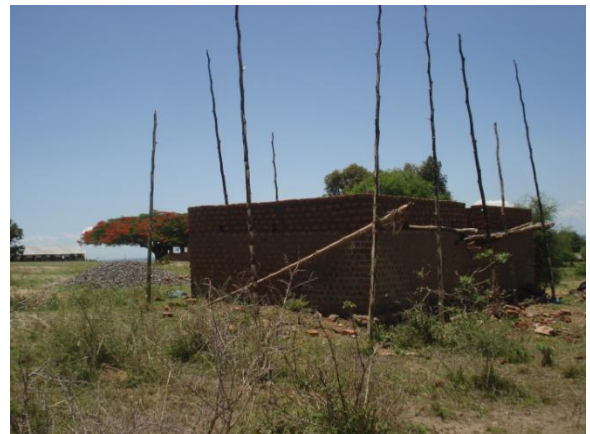
A semi permanent house being constructed by parents in Nyakagei in Panyimur Sub County.
